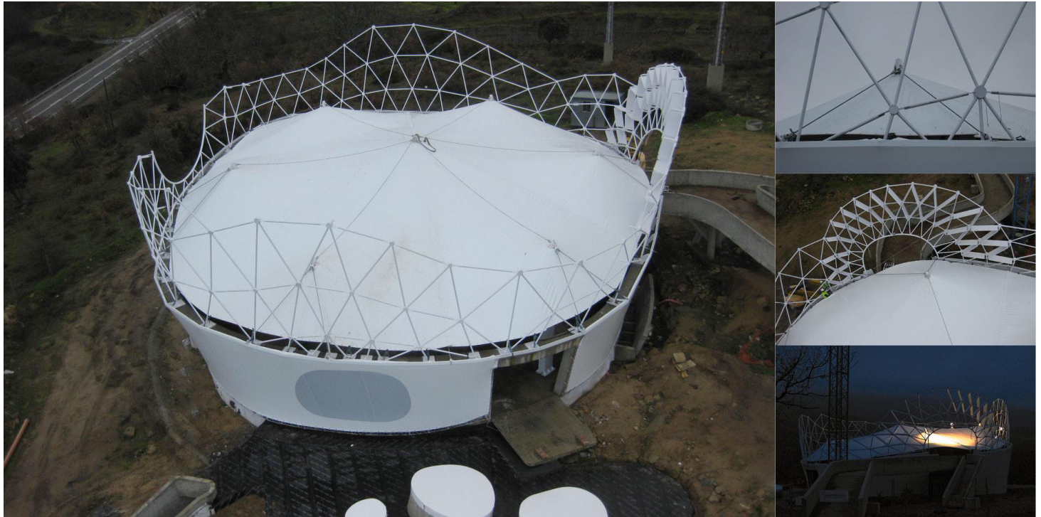
PCV membrane structure
