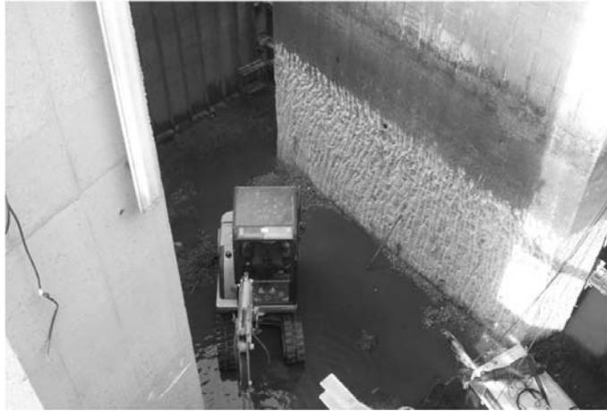
Figure 3. View of the space between two pier columns. The roughened column surface is visible.
