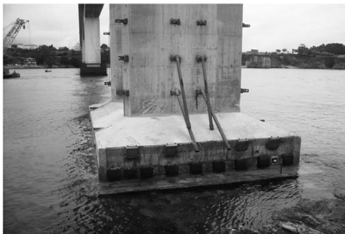
Figure 5. Final prestressed solution for foundation of the side piers. analysis of the piers
