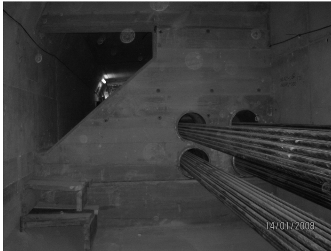
Figure 11. View of external prestressing inside the box girder crossing a diaphragm concreted in order to limit distortion of the deck.
